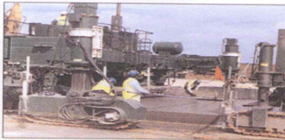
Fly ash concrete being used on East Midlands Airport taxiways (courtesy of Fitzpatrick Contracting Ltd)
